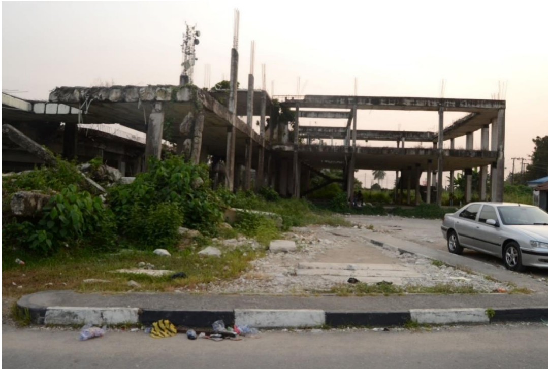
Fig. 15: An abandoned and dilapidated structure of part of UJ Esuene Stadium. Photo: Nsima Udo, 29 December 2019.
