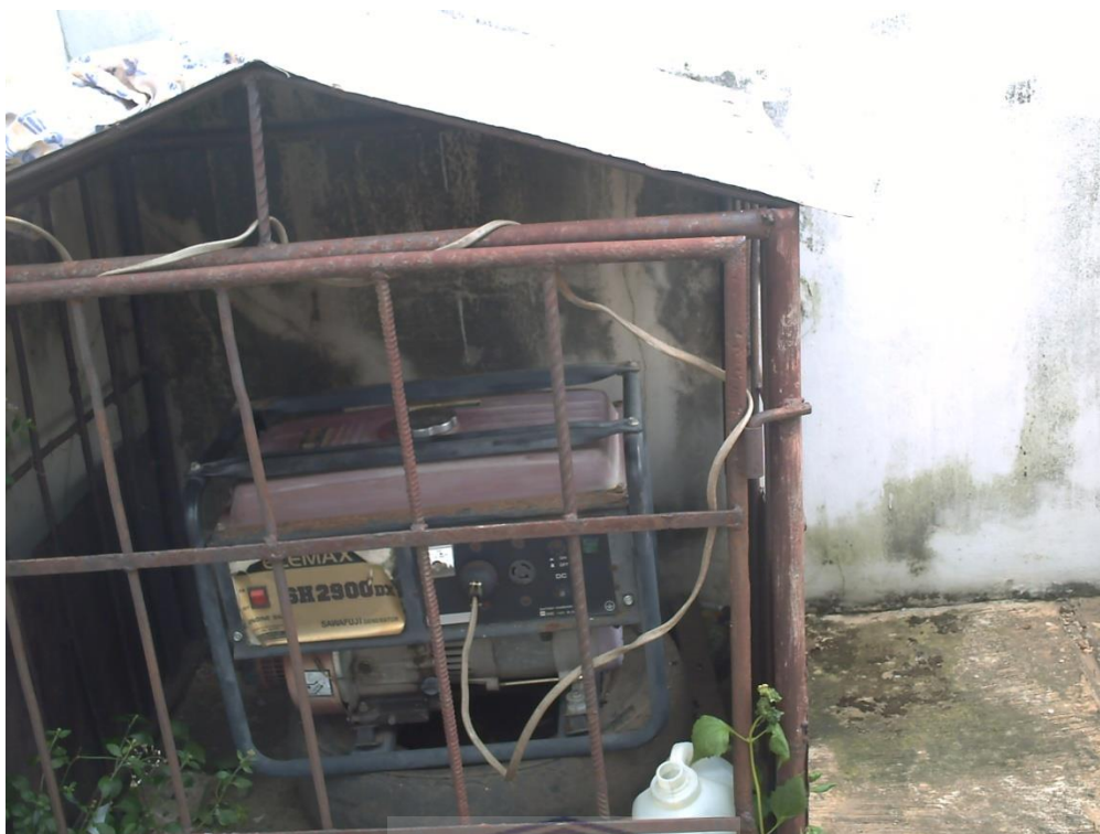
J: Electric generating set one of the PHC maternity centre
