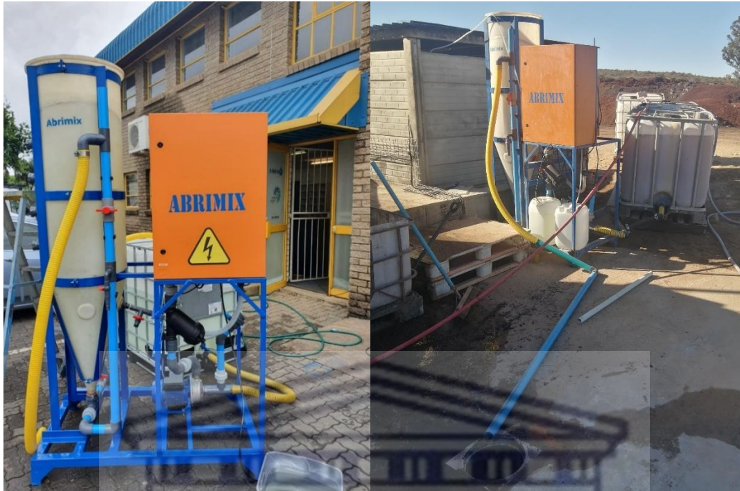
Figure 3.7. Image of Abrimix treatment plant used at Lutzville winery (2021-2022).
