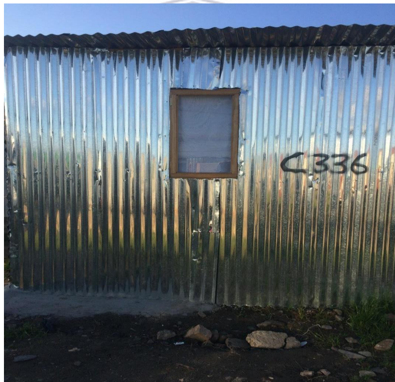
Figure 3: One of the houses marked by the residents, with a marking spray.
