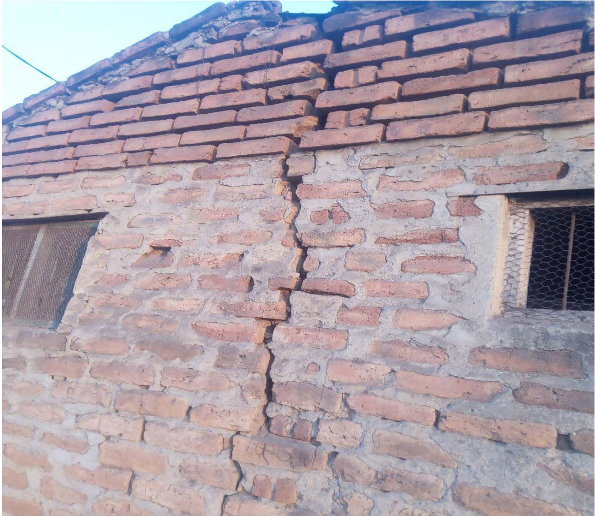
Figure 7: Cracks in the house due to mine blasting. September 2018.
