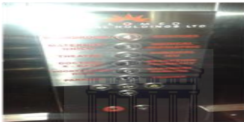
Figure 5.22: Selection Panel inside elevators at Melomed Private Hospital
