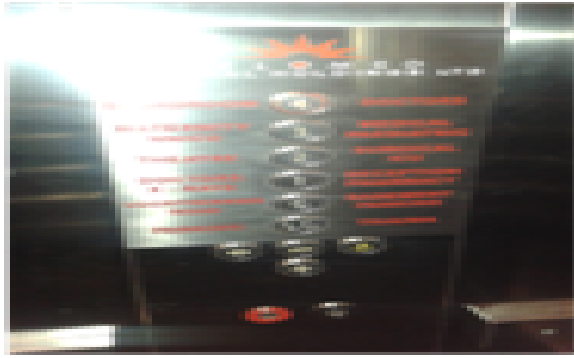
Figures 5.11: Selection panel inside elevators at Melomed Hospital
