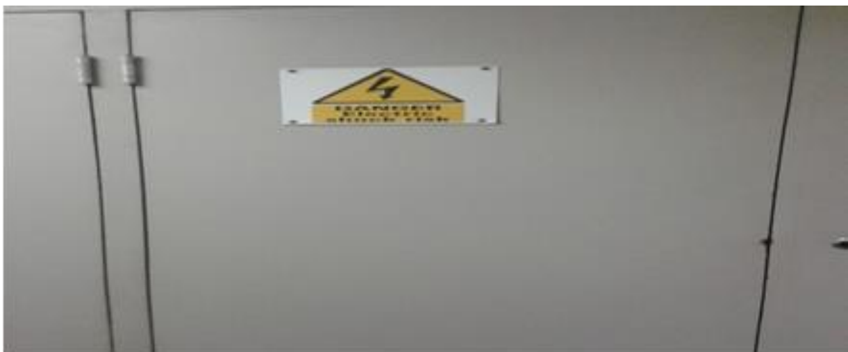
Figure 5.24: Danger warning signage placed at the door of a power control room at Melomed Hospital
