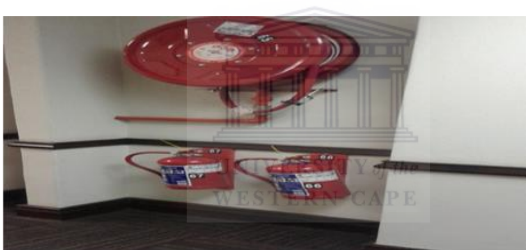
Figure 5.25: Fire response point placed in the hospital corridor at Melomed Hospital
