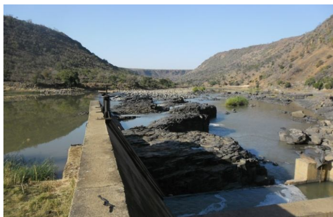
Plate 7: Wheels for opening and closing the sluice at diversion point and the stilling basin
