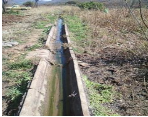
Plate 14: Leaking Canal System
